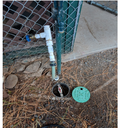
Dry Hydrant (DH) and Valve-G (in off position)
