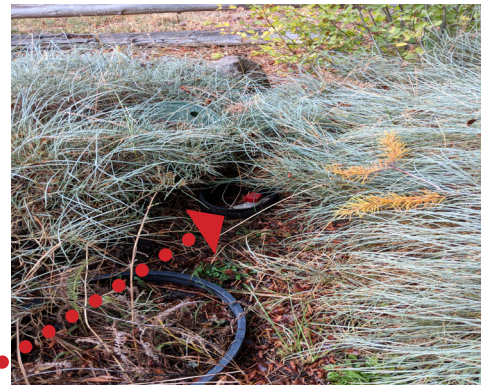
Valve B (near fence)
